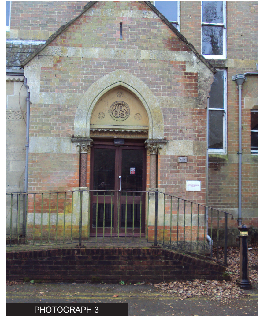
The original front entrance to 'Browfort' with raised ramp to left to provide disabled access.
